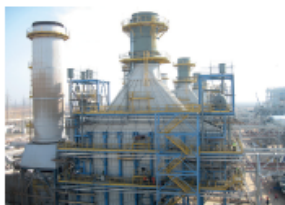
Heat Recovery Steam Generators
